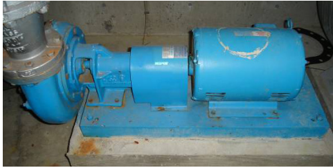
Main Pool Pump: Original Application
